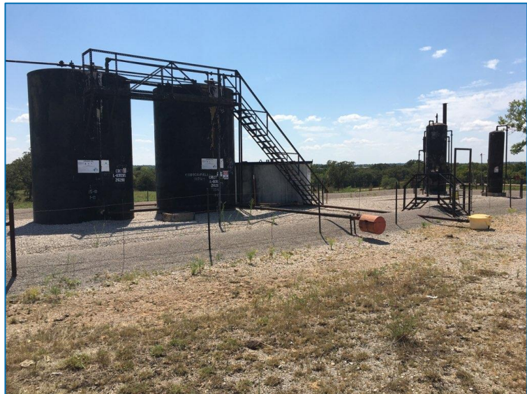
Tank battery and related production equipment, Mitchell 1-12 well, Carter County
