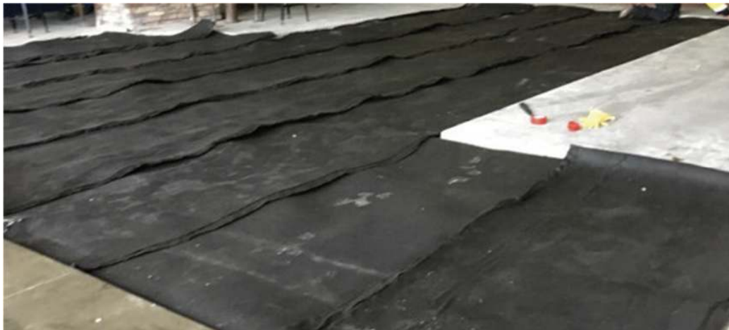
Figure 1. Interior Corridors- 3-inch-thick EdenCrete® concrete overlay on drainage system and suspended deck
