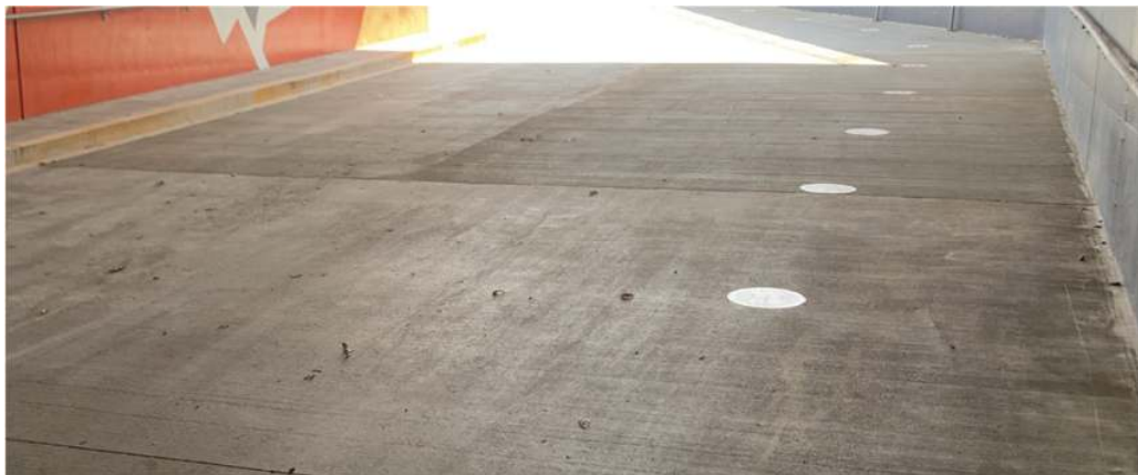
Figure 7. Freight Access Ramps- 8 inch thick slab on grade- 5000psi (35MPa) structural concrete
