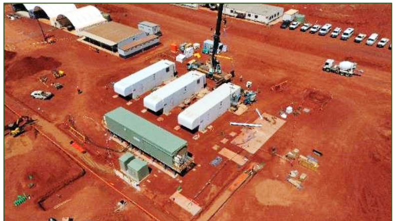
Power station equipment in place at Beyondie SOP Project
