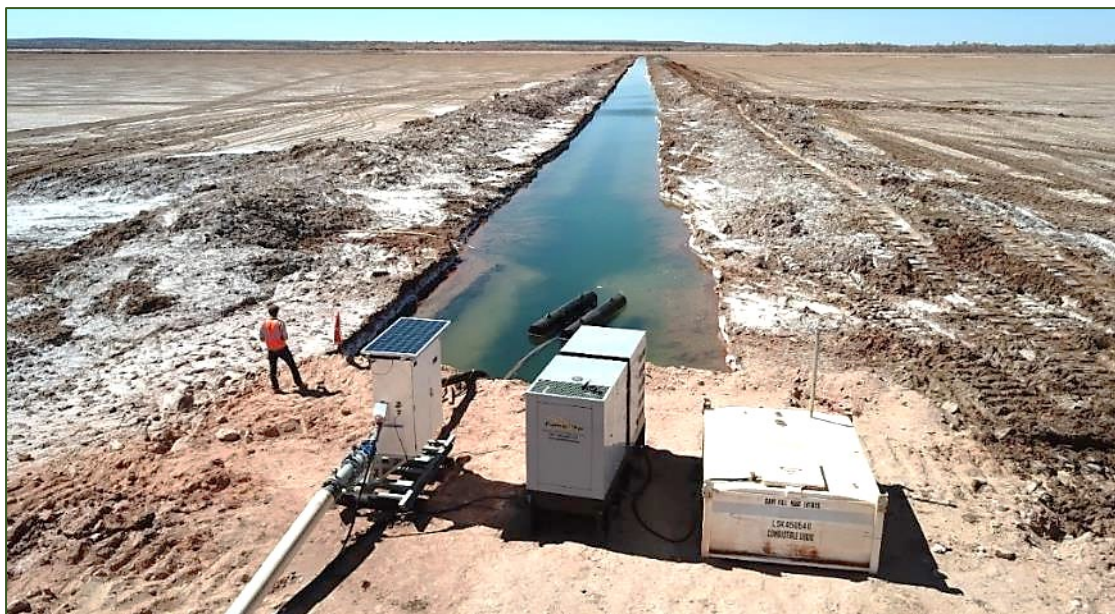
Lake Sunshine Trench Pump Station
