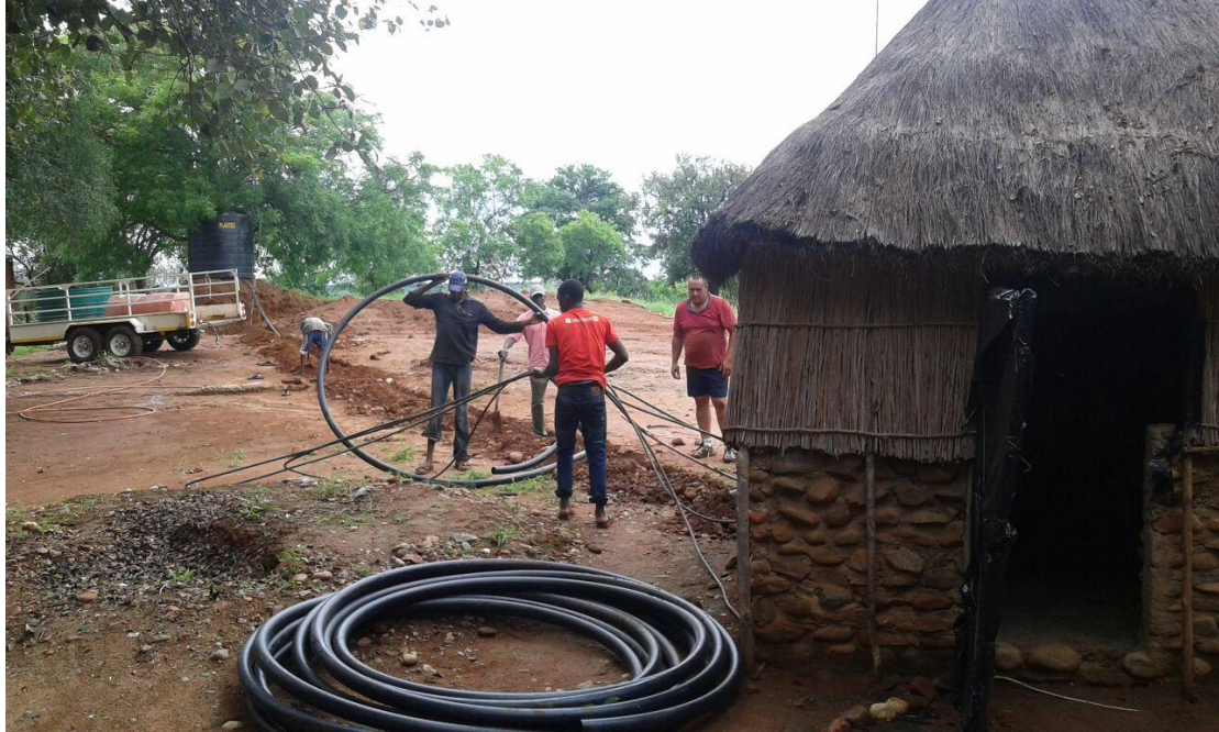
Installing water to showers and toilets at the Save River Diamonds Project camp
