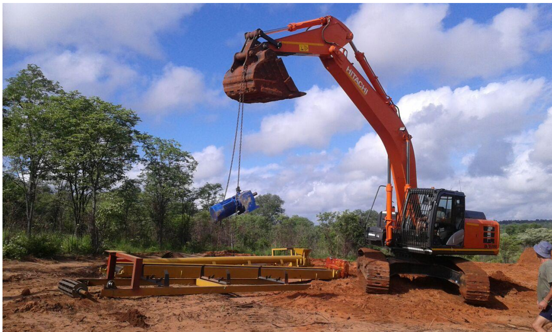
Enabling and setting up of key trial mining equipment at the Save River Diamonds Project
