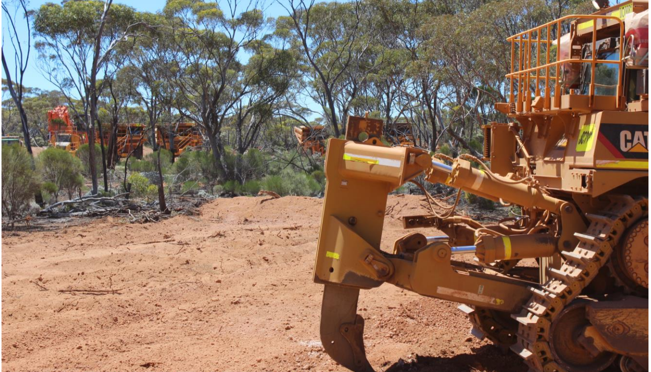
Figure 1. Start of mining at Nova – the boxcut site on Australia Day, Monday 26 th January 2014.
