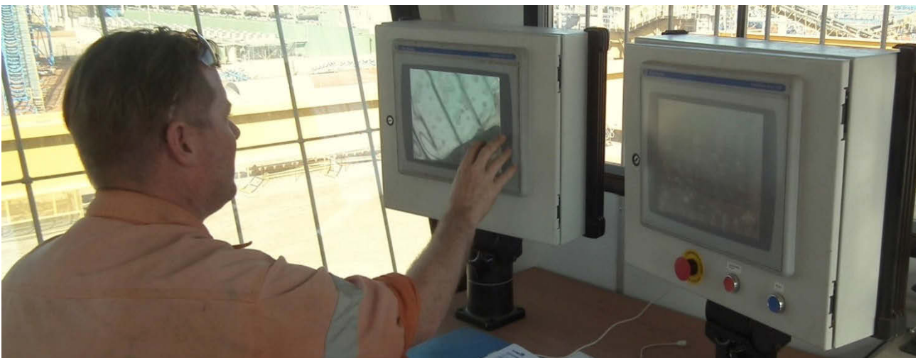
Figure 07: Crusher Operator checks settings on the Crusher Control Panel
