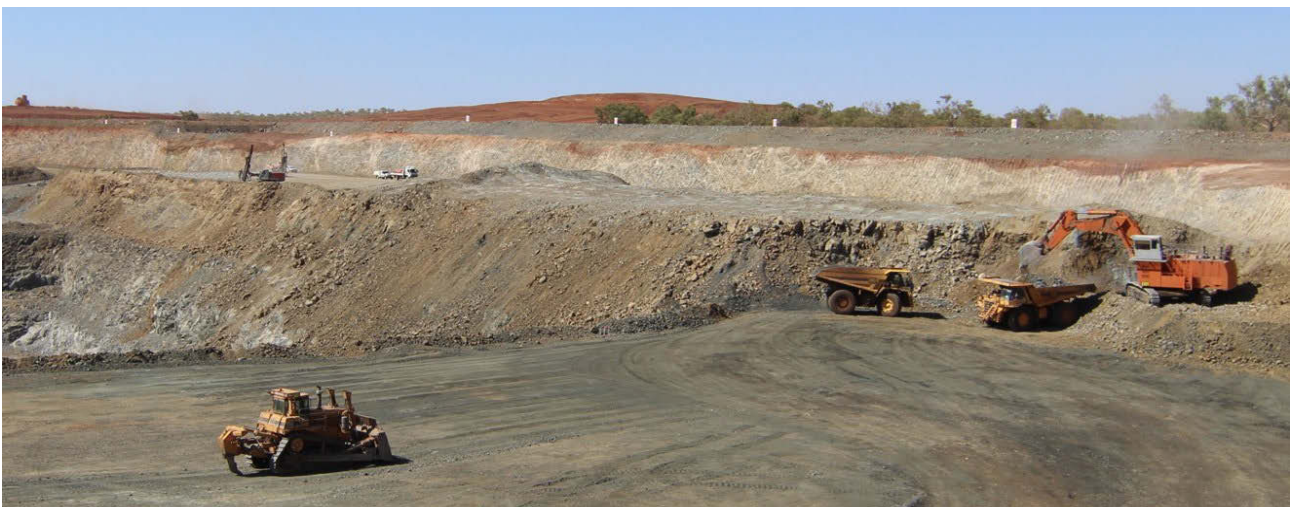
Figure 02: LM1 and LM2 Pits being mined concurrently. Blast drilling underway in background as mining continues in the foreground.
