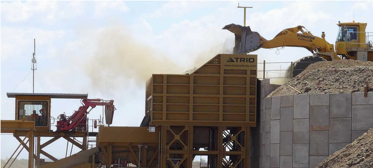
Figure 04: The crusher is fully operational, and is currently crushing and scalping native copper ore.
