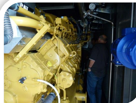
Dornesti: Gas to Power Plant
