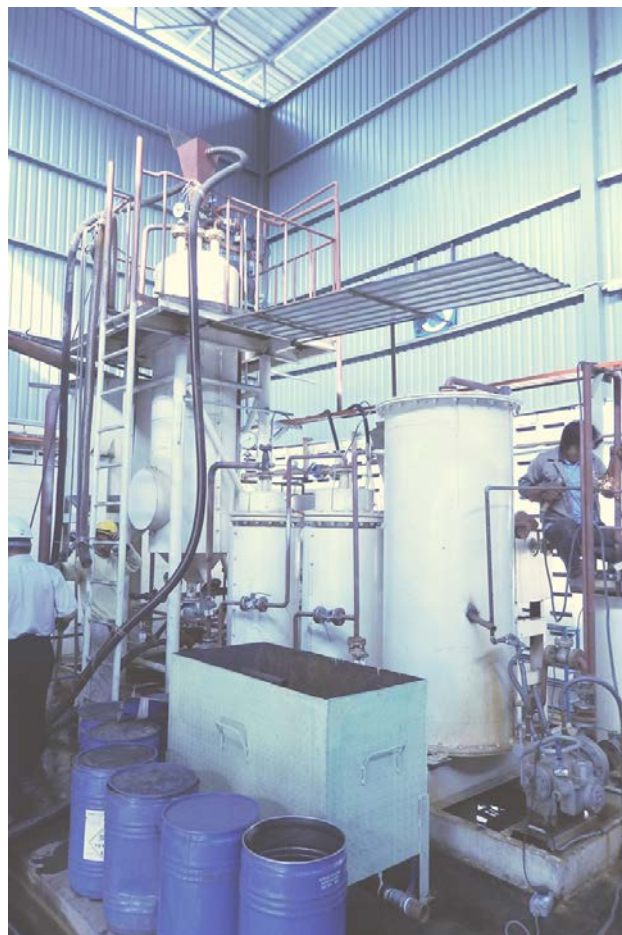
Photograph; Carbon stripping column.
