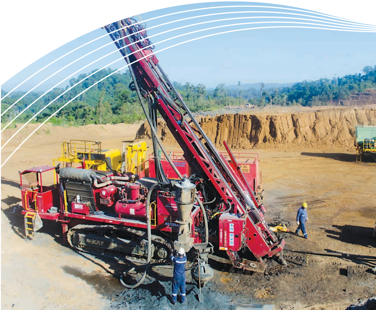
Tap AB Mirante Lode drilling with Tap AB3 open pit in background
