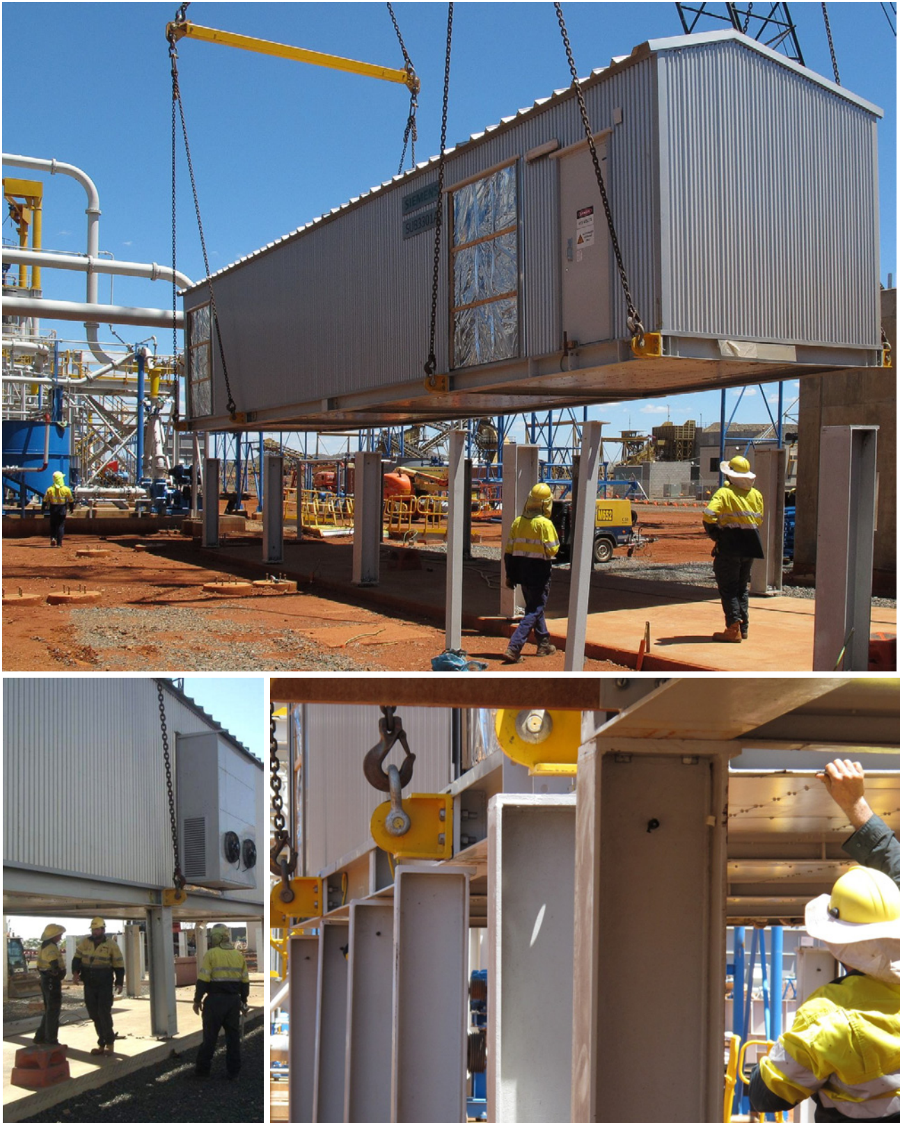
Figure 4: E-house installation at the Rocklands Process Plant clear the way for electrical cable installation which is the final major step to commissioning.
