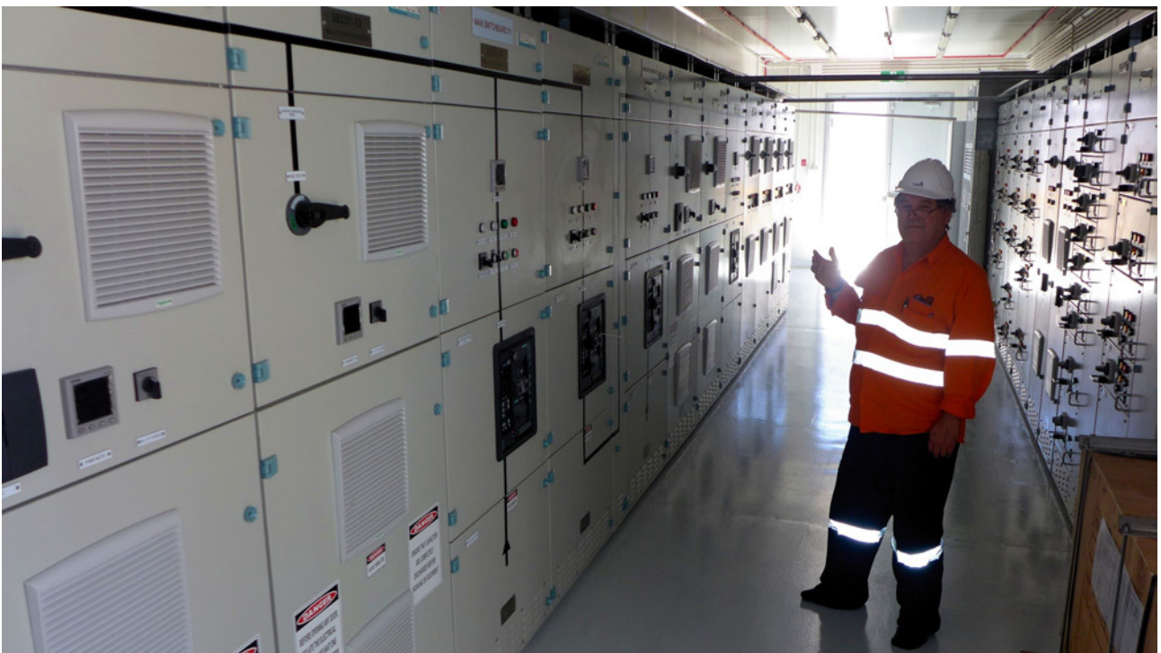
Figure 5: E-house installation at the Rocklands Process Plant (top image) and a closer look inside one of the 20 E-houses, at the various control systems and switches in one of the smaller units (bottom image).
