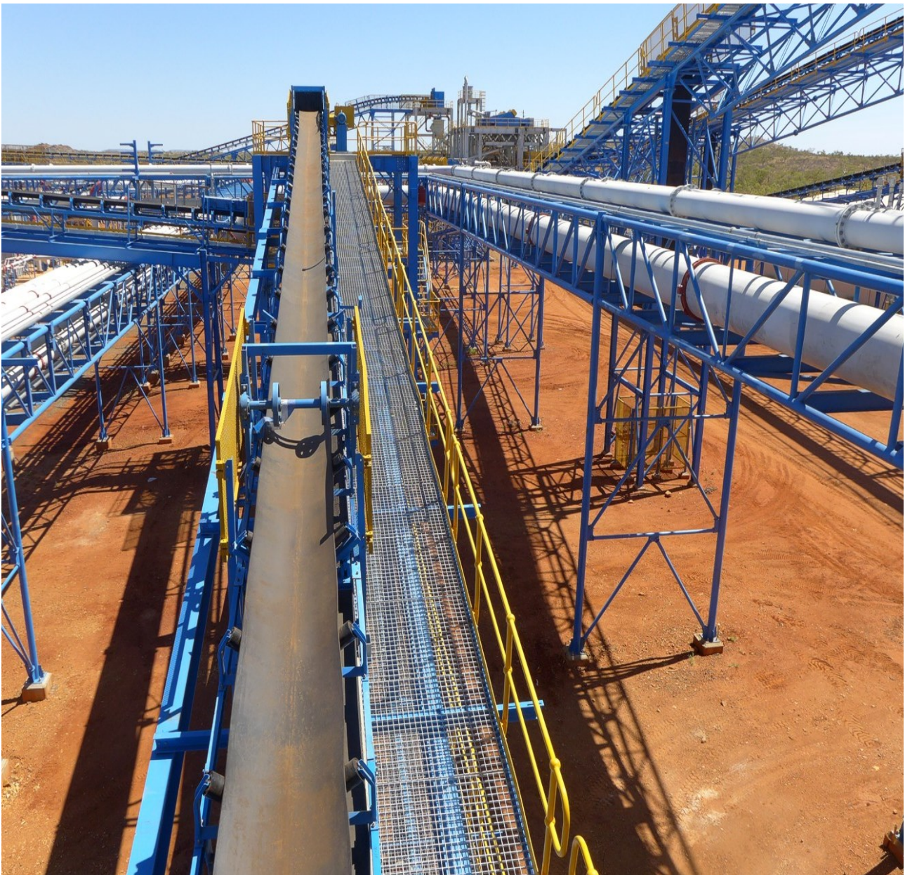
Figure 6: Rocklands Process Plant includes 15,000 tonnes of steel and more than 20,000m 3 of re-enforced concrete. Components for the project were delivered in 33 shiploads from around the globe including China, Japan and Germany.
