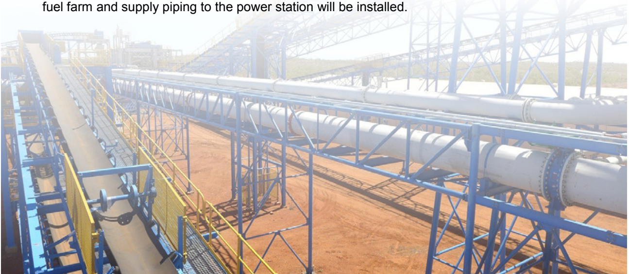
Figure 2: The Process Plant includes over 3,000m of conveyors and 18,000m of piping - now completed.
