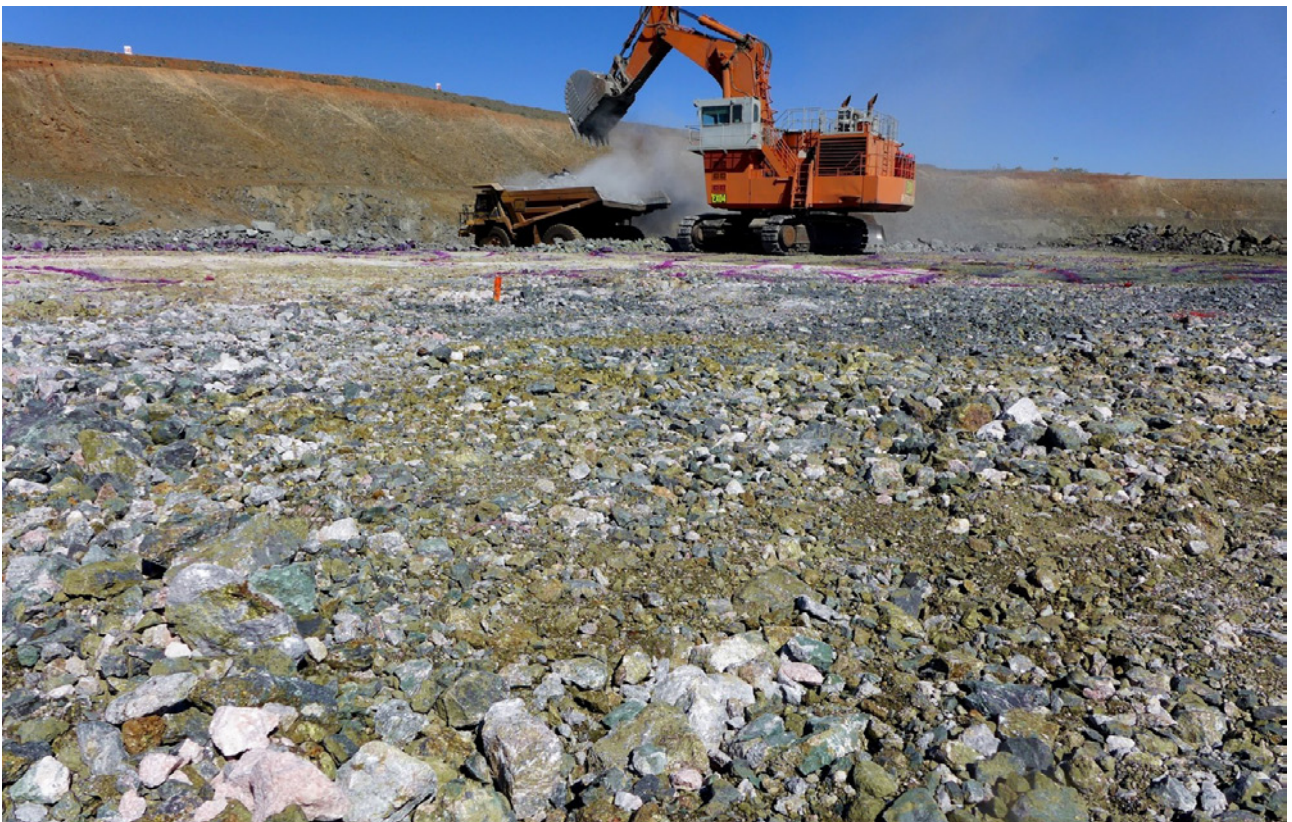
Figure 13: LM2 Pit floor at RL195 - approximately 60m wide ore zone of very high-grade primary copper ore (chalcopyrite, bornite, chalcocite), cobalt ore (pyrite) and magnetite, strewn across the pit floor.
