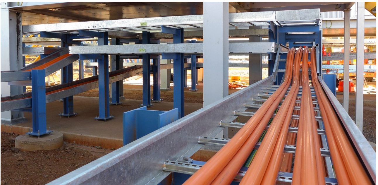
Figure 4: Cable support trays being stalled along the side of the Gravity Jig building (top image); and cable-trays and cables leading to one of the 20 E-houses at the Process Plant that will control the electrical systems.
