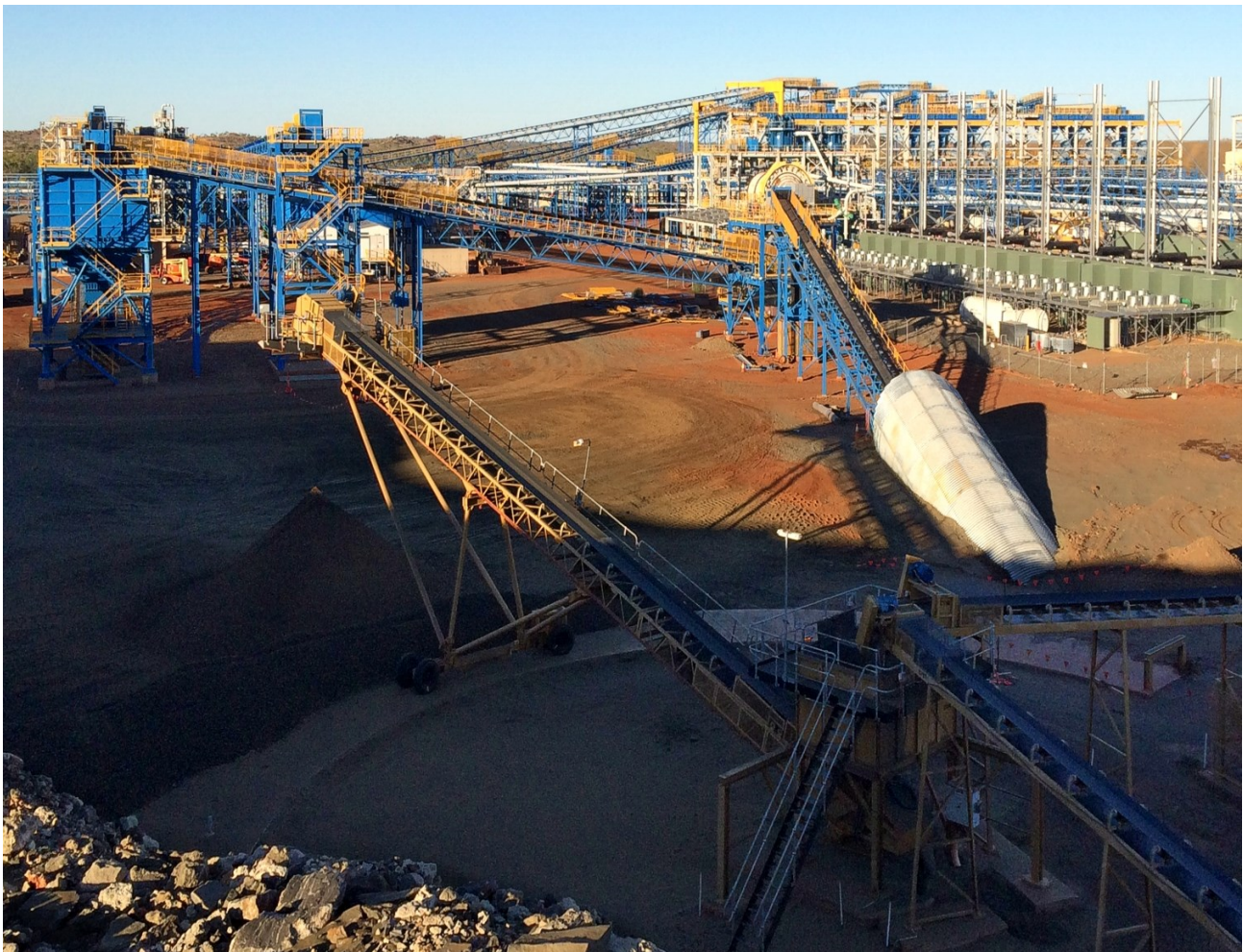
Figure 17: The crushing circuit is currently running 24 hours per day to remove oversize native copper (+40mm) prior to commencement of processing in main mineral processing plant that is currently under construction. The yellow conveyor left foreground radial stacks crushed ore (-40mm) prior to loading into the HPGR tunnel (white tunnel structure - centre foreground) for transfer to the HPGR and processing through the plant.
