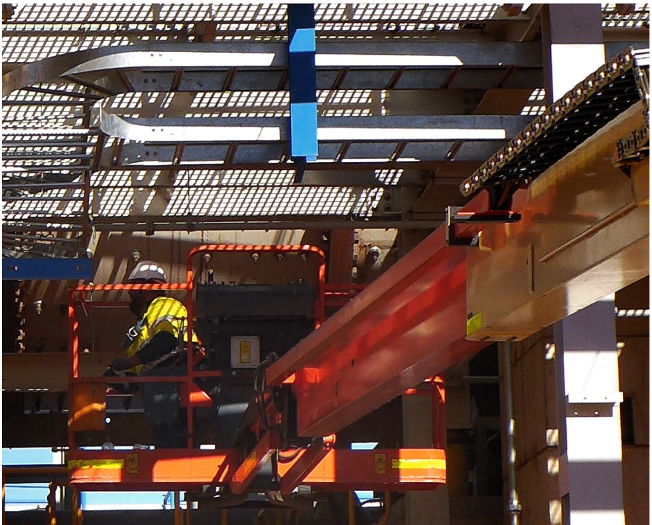
Figure 7: Installation of the many cable support structures is timed for completion prior to running cable.
