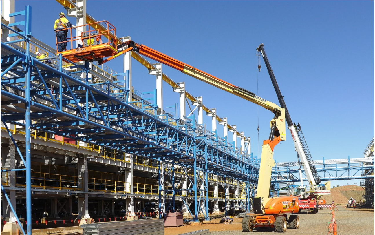
Figure 5: Earthing cable (top left), cable-tray installation at the Spirals building (top right) and support structure and cable-trays being installed along the Gravity Jig building (bottom image)
