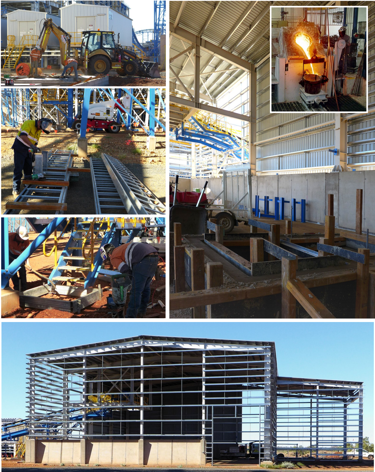
Figure 10: Excavation for cabling at one 20 E-houses (top left); assembly of cable trays (middle left); pouring concrete landing (bottom left); construction underway at new copper casting plant (top right); and native copper storage shed being clad (bottom)
