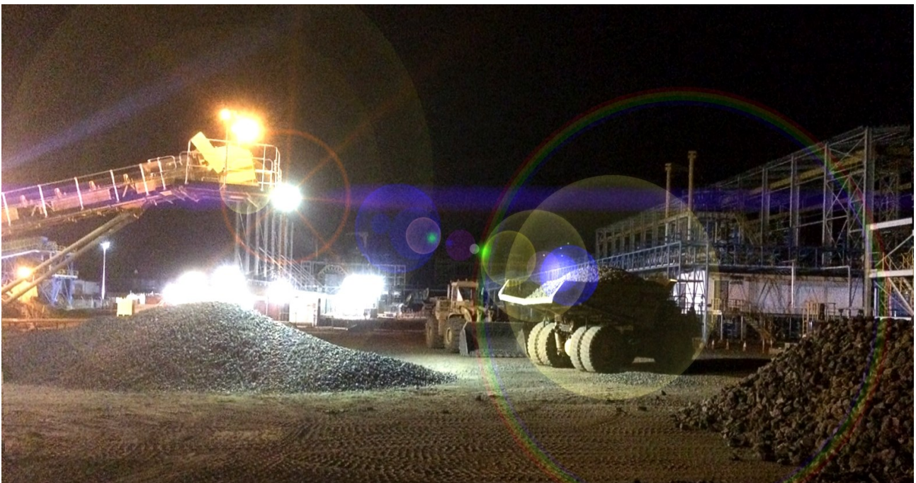
Figure 18: Primary Crusher feed bin being inspected during maintenance periods (top) and 24-hour crushing is adding significantly to crushed ore stockpiles (below).
