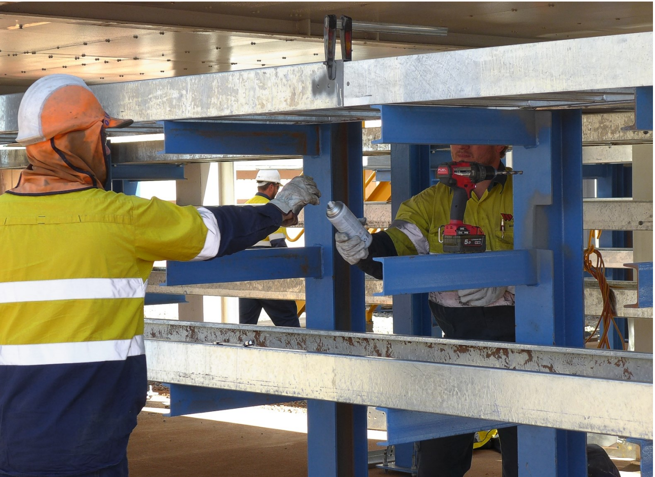
Figure 6: Installation of the many cable support structures and trays is timed for completion prior to running cable.
