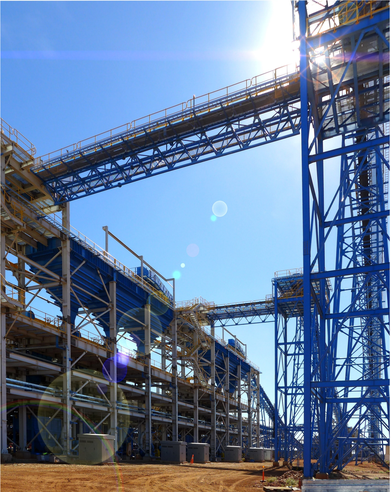
Figure 8: Rocklands Process Plant includes 15,000 tonnes of steel and more than 20,000m 3 of re-enforced concrete. Components for the project were delivered in 33 shiploads from around the globe including China, Japan and Germany.
