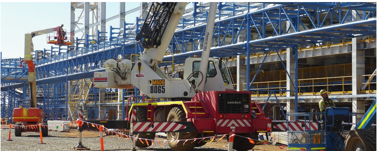
Figure 2: Cables pulled to E-house termination points (above) and cable-trays being installed at the Gravity Jig building.
