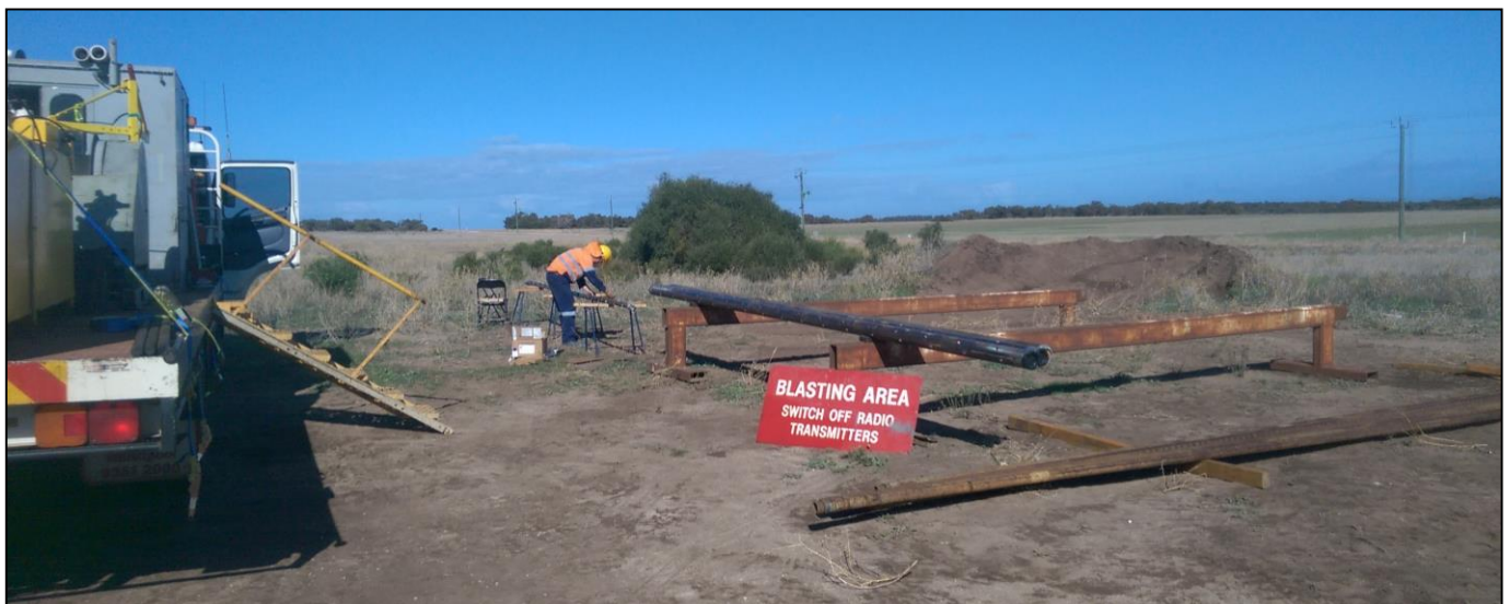
Preparation of perforating guns (above left), inserting guns and detonators into gun carriers (above right) and Westlog wireline unit and gun carriers (x2) and safety joint on racks (bottom)
