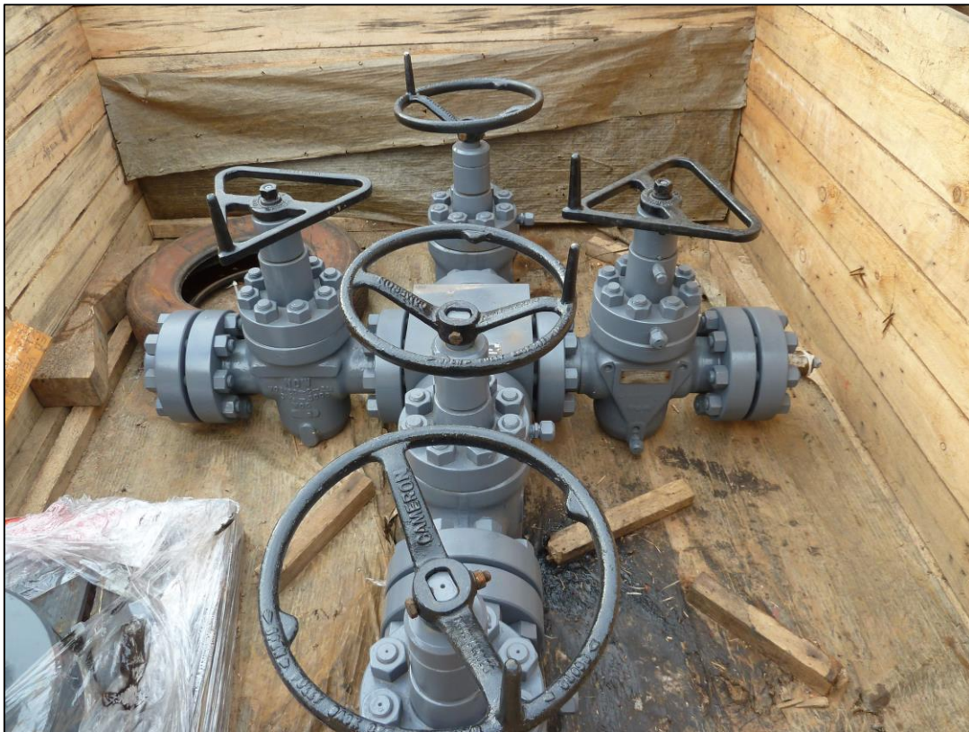
View looking from rig floor south towards flow back tanks and completion jewellery to the left (above) and Production Christmas Tree to be nipped up to wellhead in coming days after nipping down of BOP
