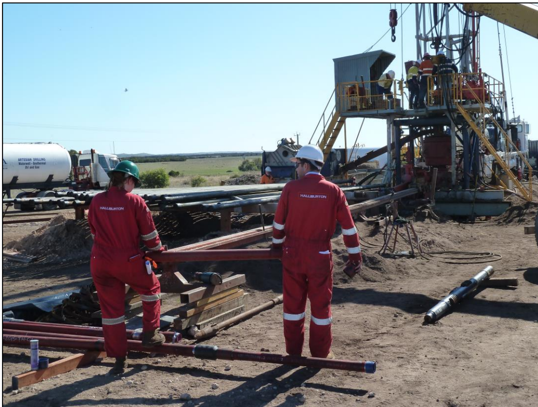
DCA, Key and Halliburton crew preparing to run production completion (above) and view looking north of rig floor (below) preparing to run in hole Westlog TCP guns and Halliburton completion equipment (foreground)
