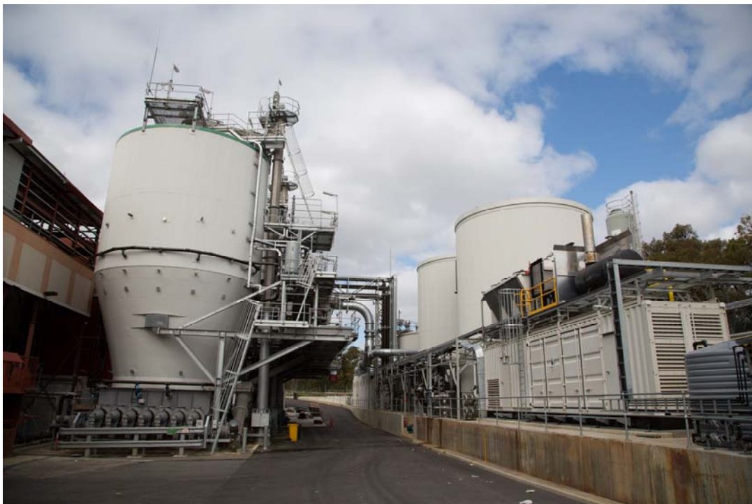
Figure 1: DiCOM™ bioconversion vessel (left) and the gas fired combined heat and power (CHP) generation unit for the production of renewable electricity and heat (right).
