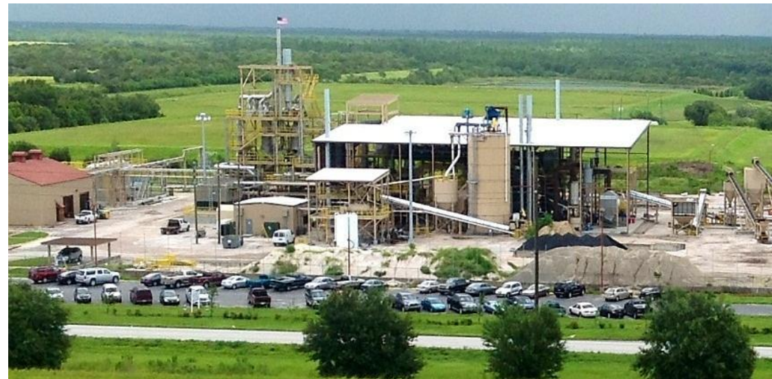
JDCPhosphate IHP Demonstration Plant – Florida
