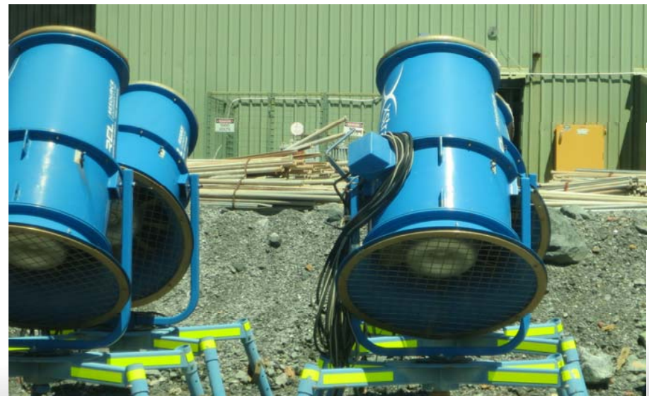
Water evaporation fans
