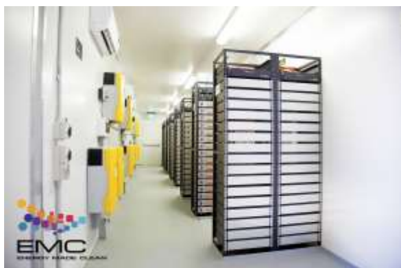
Battery system (photo courtesy of Energy Made Clean)
