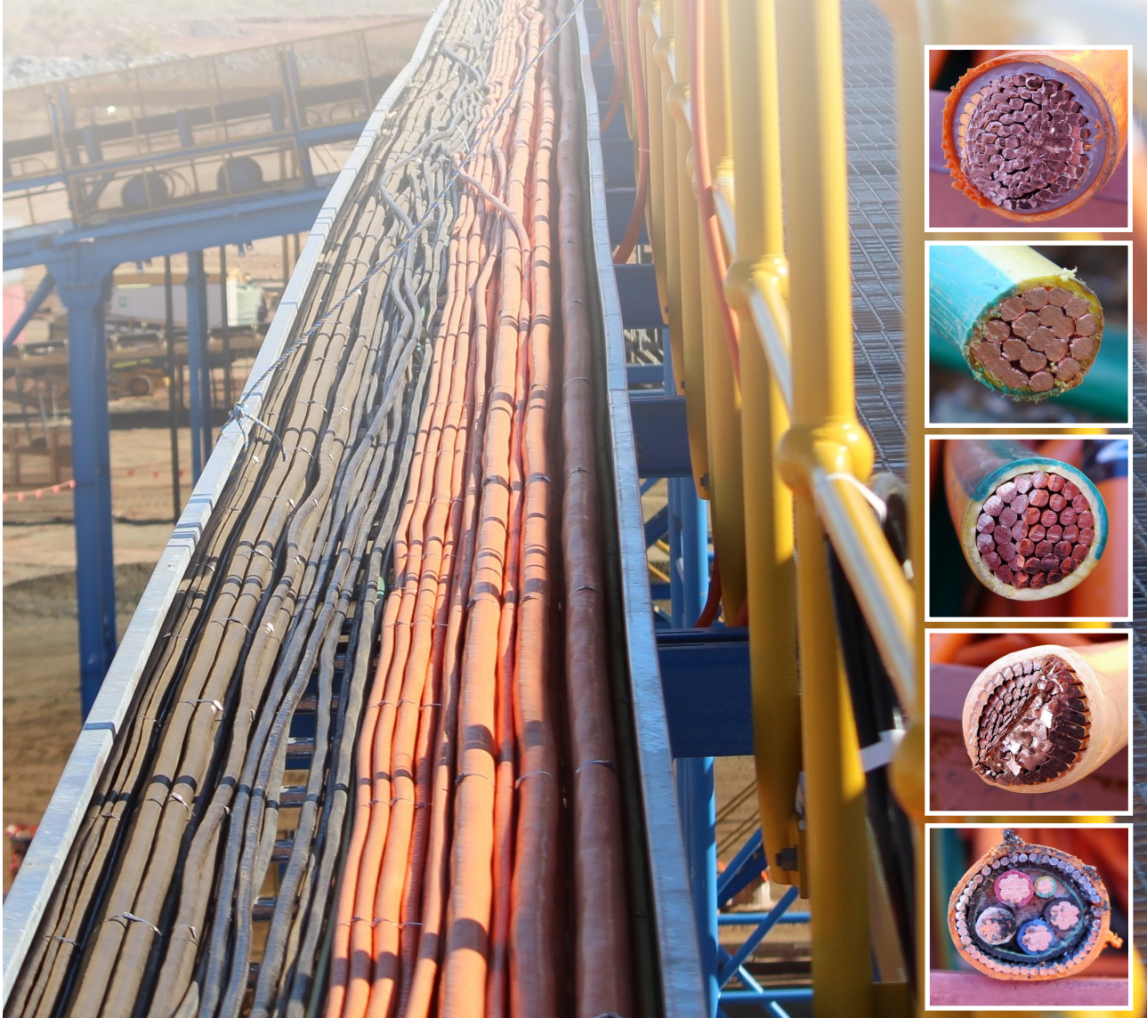
Figure 2: Cable trays run the length of the conveyor (inset shows examples of different cable types).
