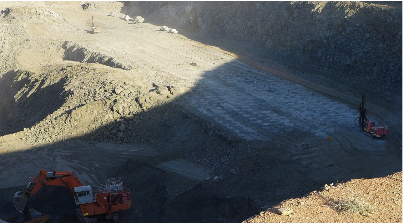
Figure 14: Mining in LM2 Pit (top image) whilst blast-hole drilling prepares for the next blast (bottom)
