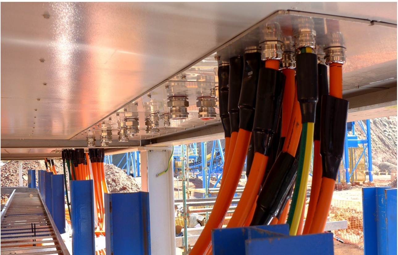
Figure 1: Electrical cable connected to one of the projects 20 E-houses.
