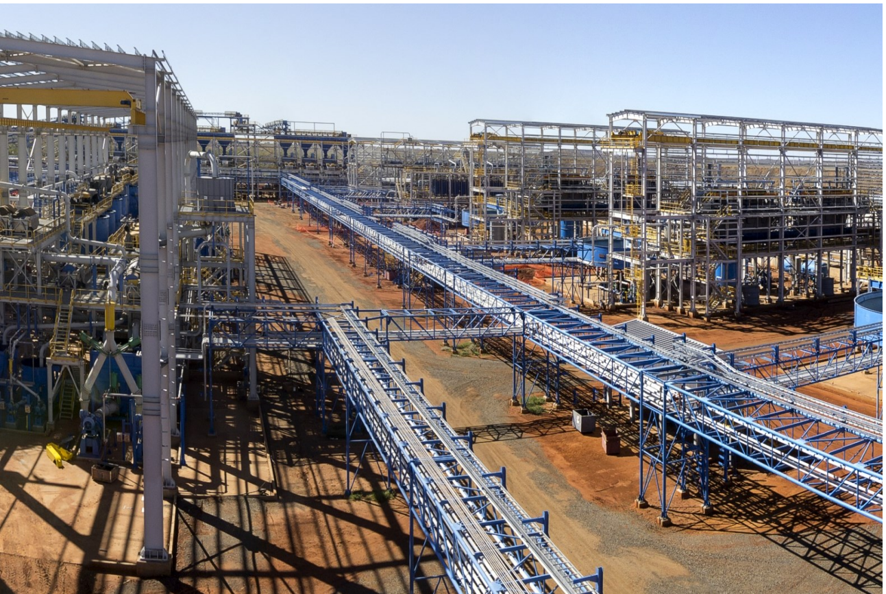
Figure 9: Various views of the Process Plant.
