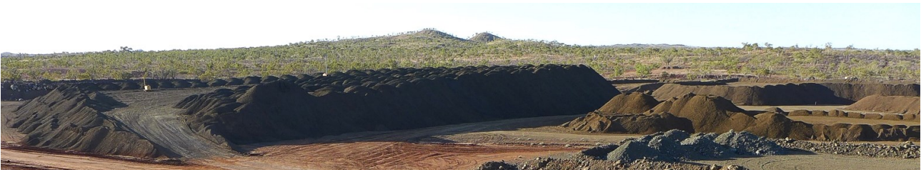
Figure 18: Crushing circuit with ROM in background (top image); and crushed ore stockpiles are now well over 300,00 tonnes (bottom)
