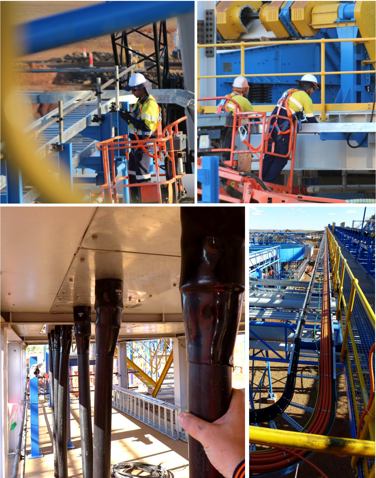
Figure 4: Cable support trays being installed (top image); and large diameter cables connected to one of the 20 E-houses.
