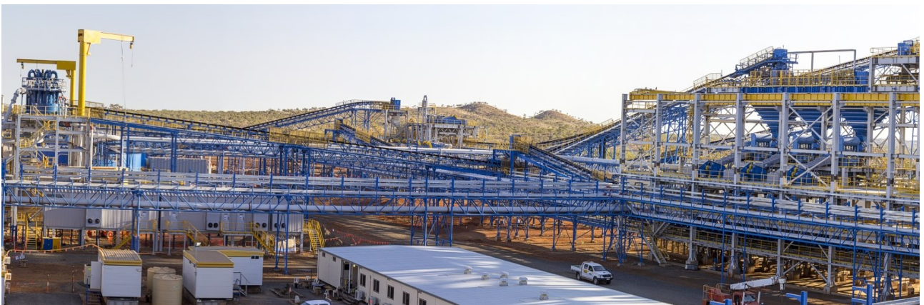
Figure 8: Rocklands Process Plant includes 15,000 tonnes of steel and more than 20,000m 3 of re-enforced concrete. Components for the project were delivered in 33 shiploads from around the globe including China, Japan and Germany.
