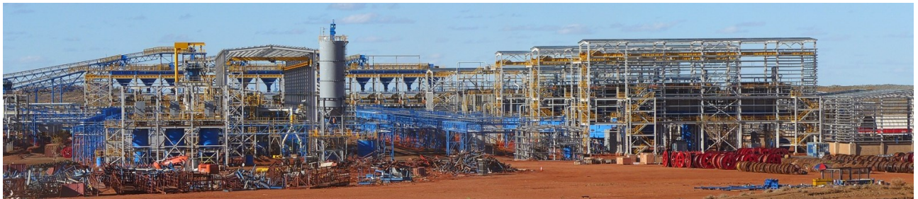
Figure 12: Various views of the Process Plant.
