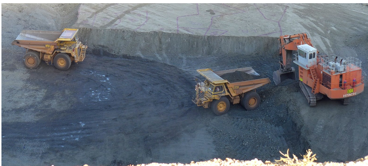
Figure 13: Pit scheduling schematic (top image) and mining in supergene ore at the north of the LM2 Pit (bottom)
