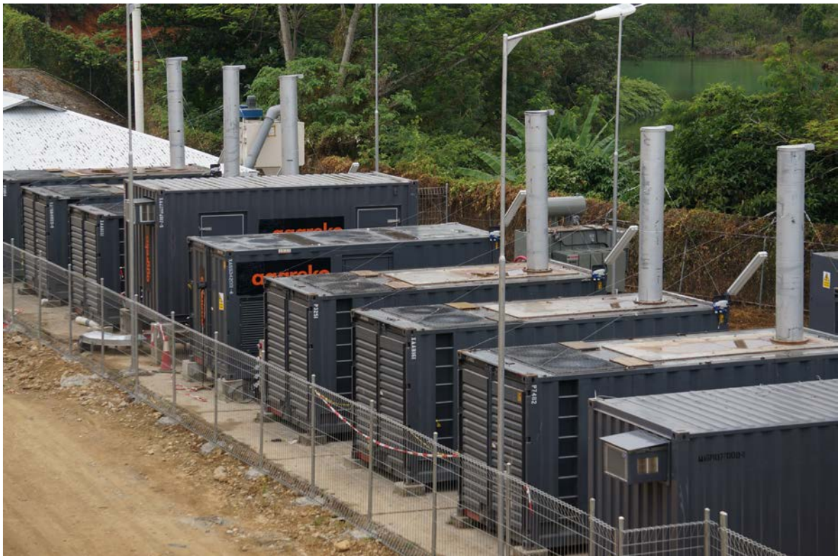
Figure 3. Power station at the CIL plant
