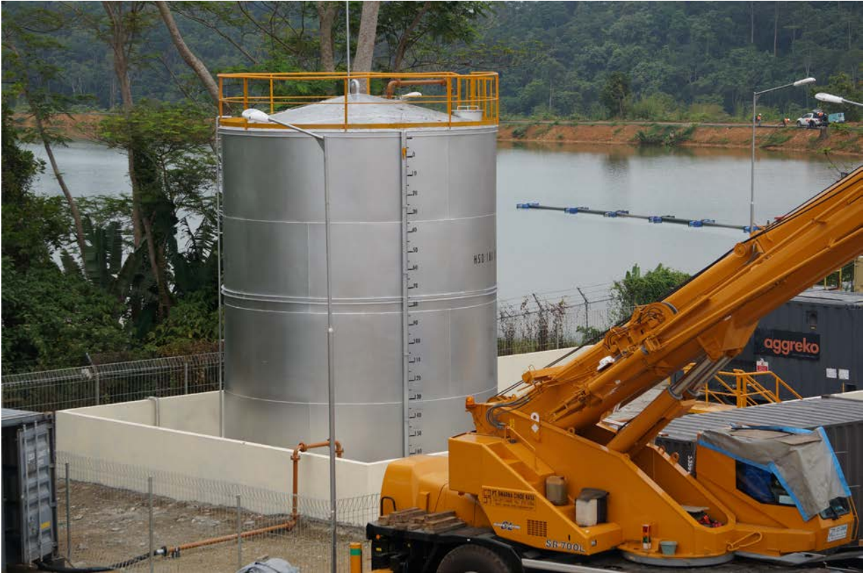
Figure 4. Fuel storage area at the CIL plant
