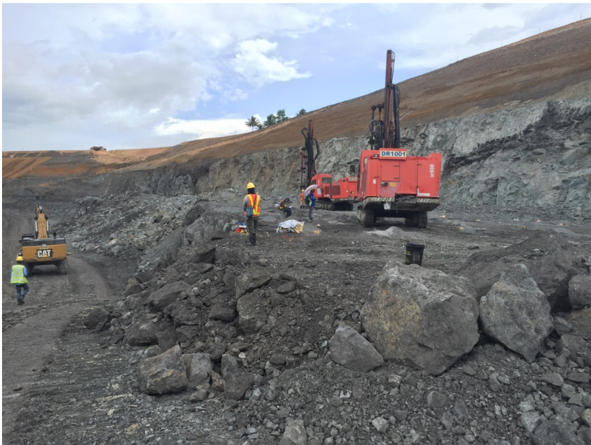
Figure 2: Mining activities at the Western wall cut-back in the Siana open pit
