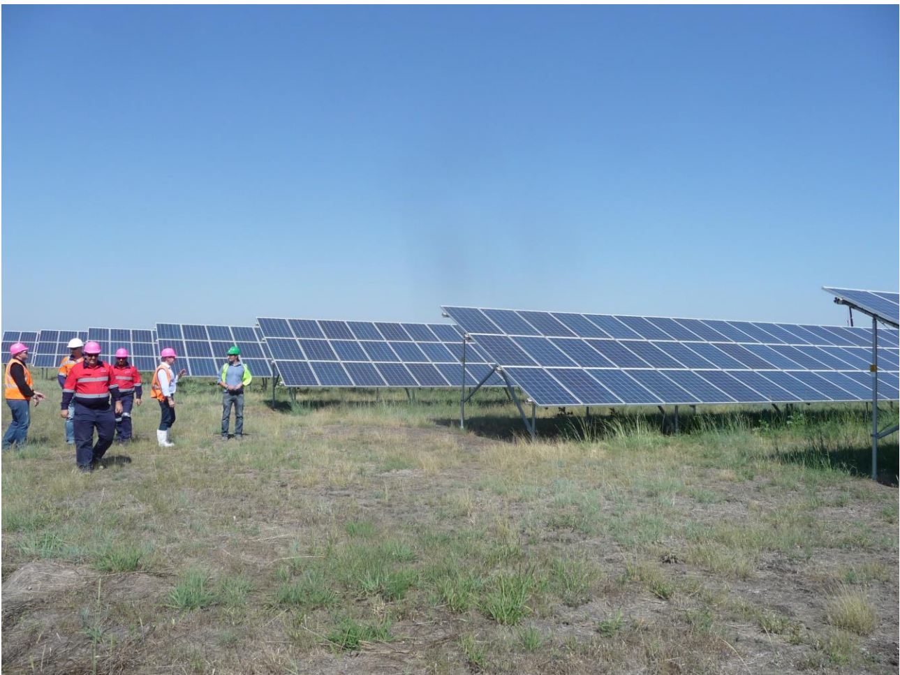
Solea AG Mine site Solar Power installation (South Africa)
