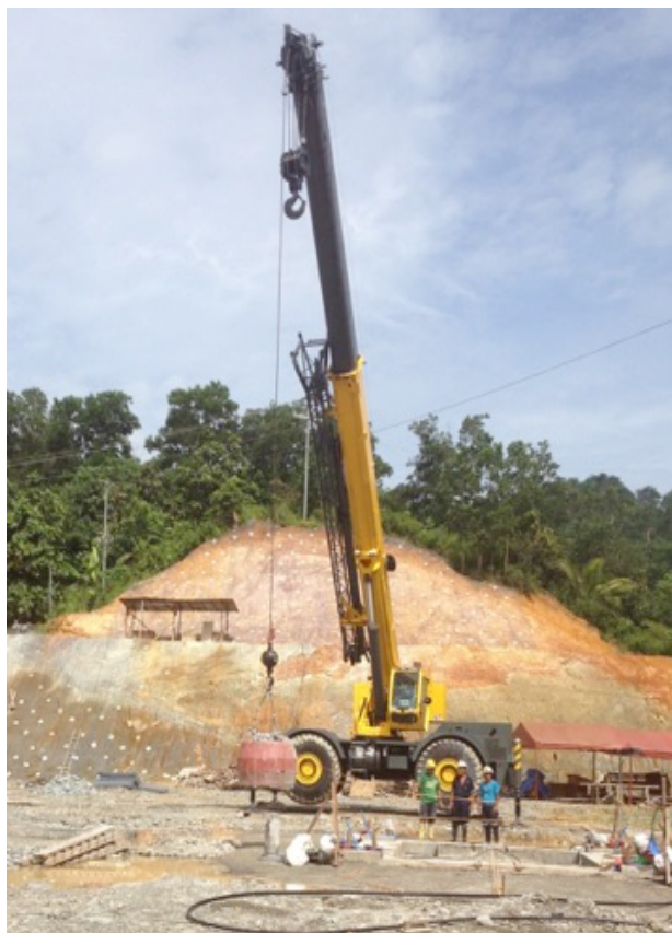
Photo 1. Service Shaft Collar showing crane and kibble used for the blind sinking.
