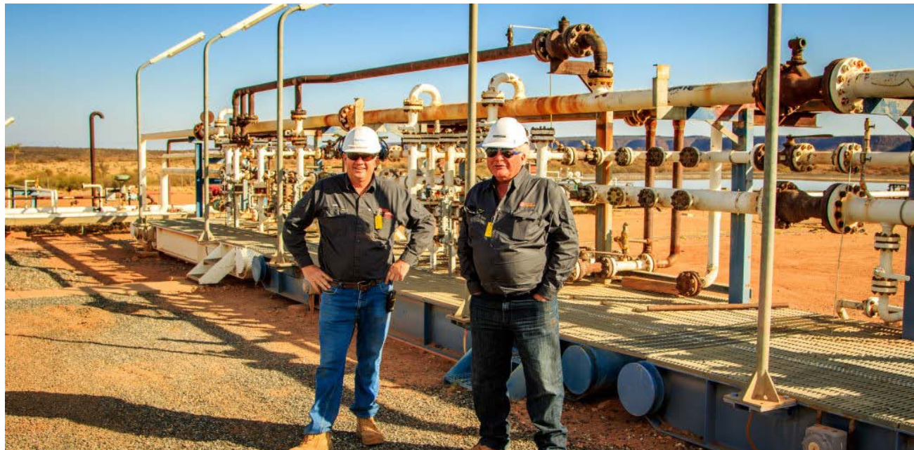
(Top left) Figure 5: Portion of the central processing facilities at Mereenie. (Top right) Figure 6: Maintenance of three phase separator (oil, water, gas) at Mereenie. (Middle left) Figure 7: Road trains in route to transport Mereenie crude oil to Port Bonython, SA. Figure 8: Cameron Crawford (right) Central General Manager Operations and Dan Casey (left) Production Supervisor inspect field gathering system at Mereenie. (Bottom) Figure 9: Paul McClelland, Area Superintendent and Andrew Whittle, recently retired Chairman of Central Petroleum standing in front of Mereenie's production manifold.
