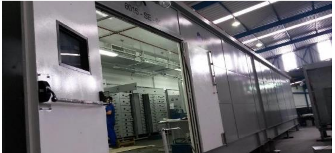
Flotation area electrical installation is simplified by the use/delivery of pre-wired Motor Control Centers
