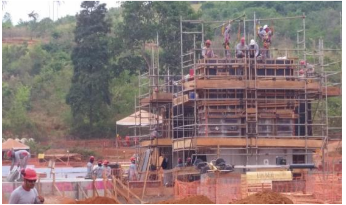
Installation of the Ball Mill concrete foundation represents the most complex item of civil work of the project. This activity has now reached the trunnion pedestal elevations where precision is paramount
