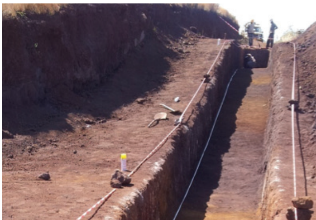
Figure 4: One of the trenches at Ngualla excavated for the pilot plant bulk sample
