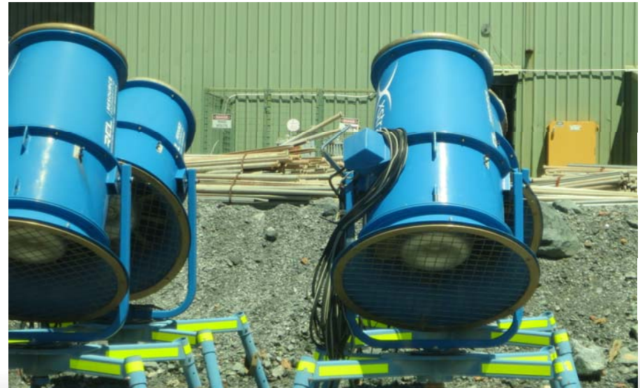
Water evaporation fans
