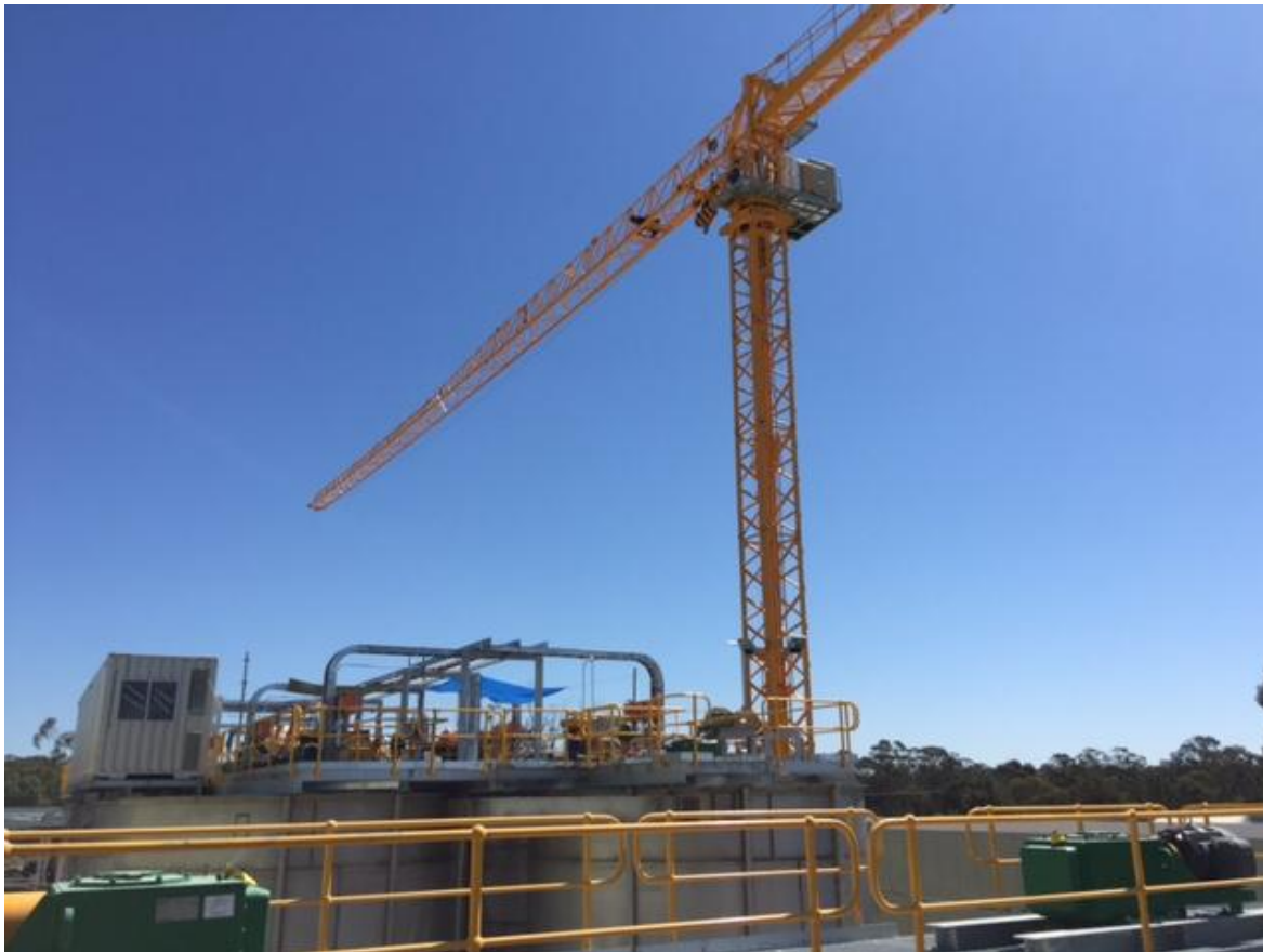
Photograph 2: The new CIL Gold and Silver process plant
