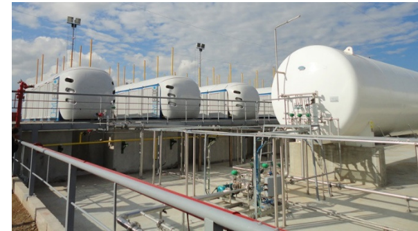
Cryogenic plants for converting natural gas
