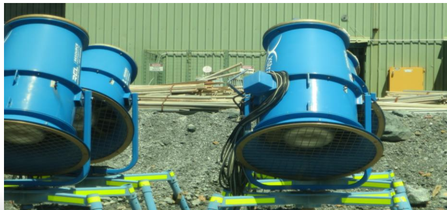
Water evaporation fans
