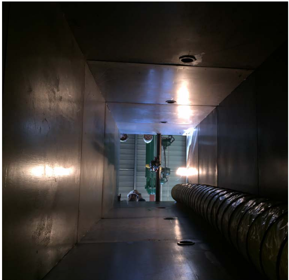
View up the Pandeniya shaft after running in liner boxes and ventilation system
