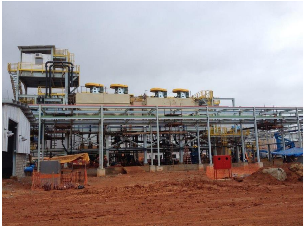
Installed flotation cells with plant control room overlooking cells
