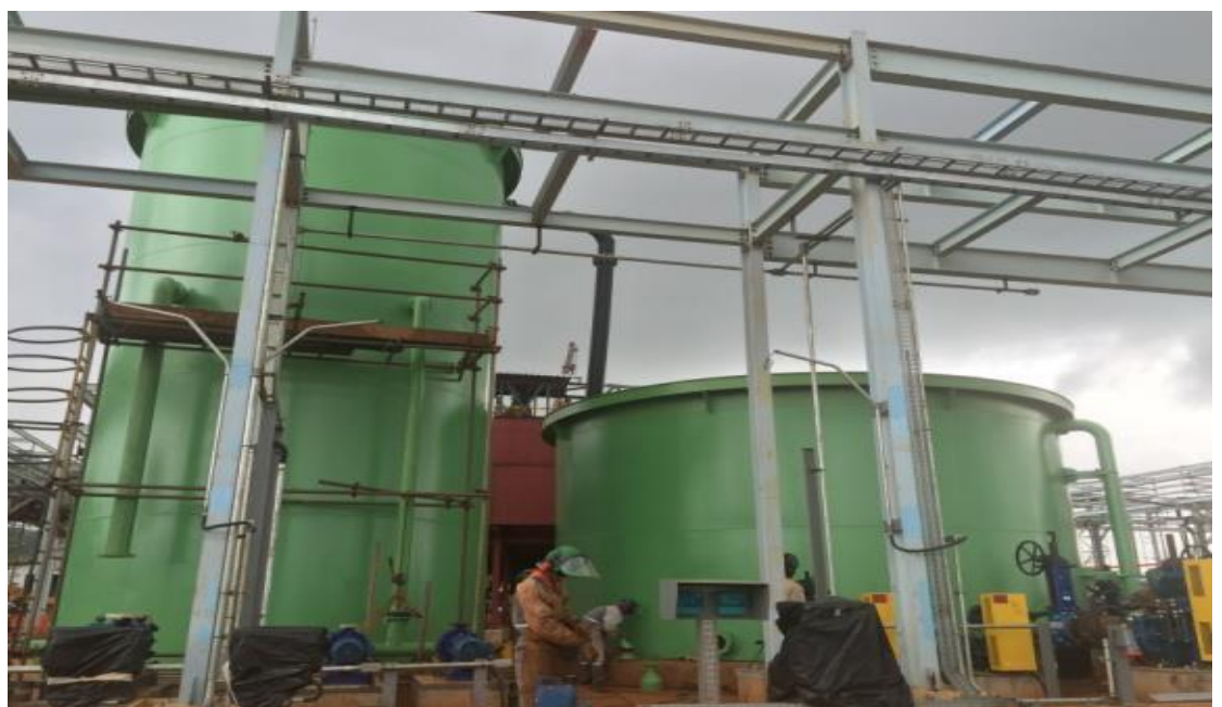
Process and raw water tanks
