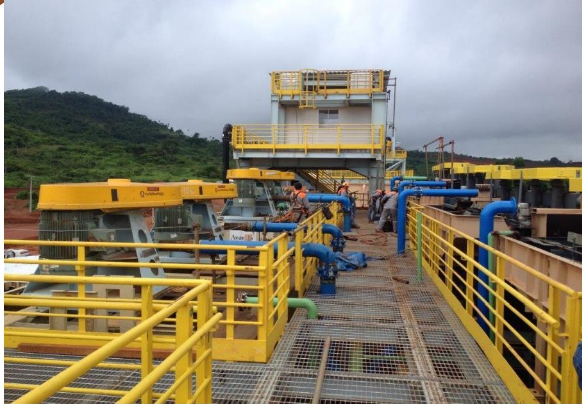
Finalising flotation cells mechanical erection activities with plant control room in background
