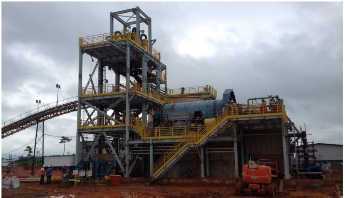
Ball mill, feed conveyor and hydrocyclones now installed.
