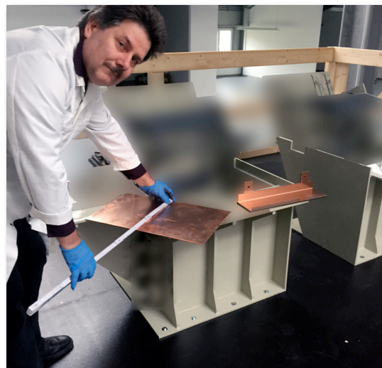
Figure 5. 2 x 50kg feed exfoliation cells being installed. Note: some components intentionally blurred to protect IP.
