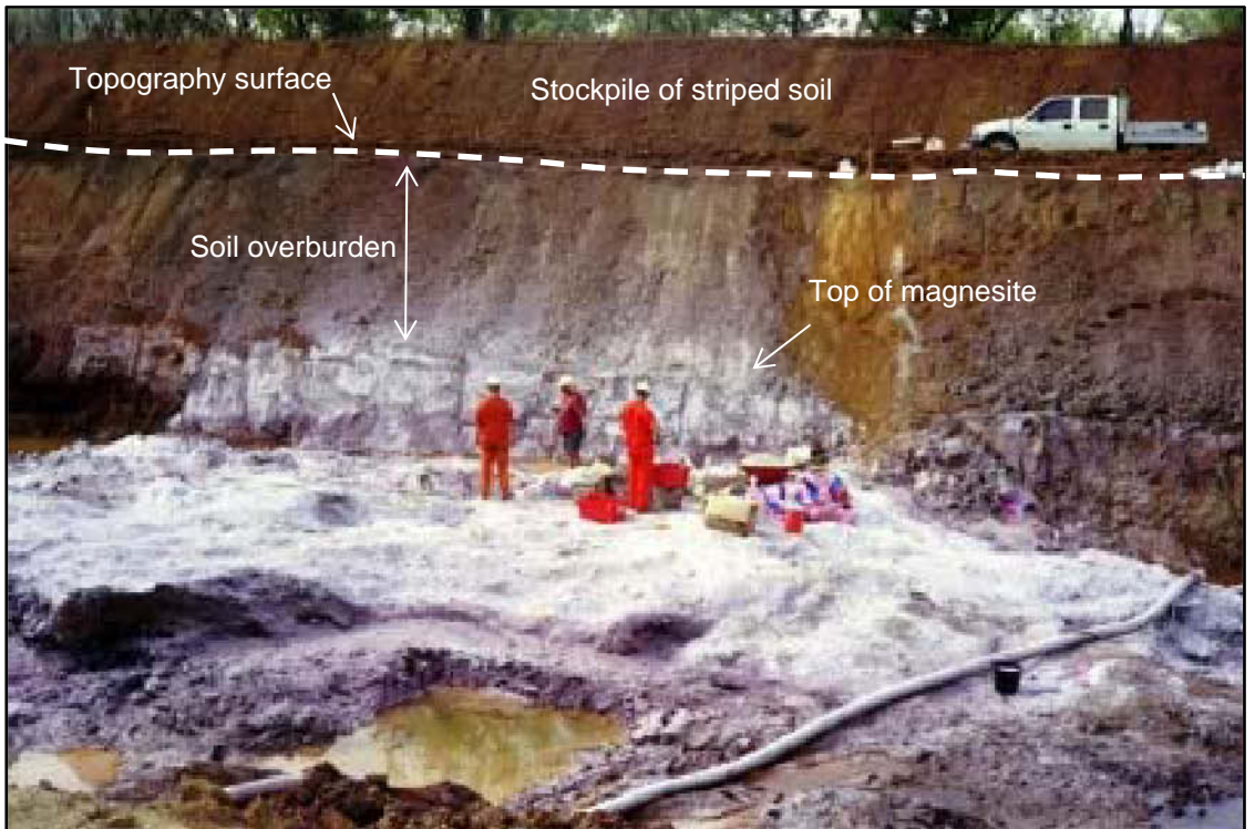
Figure 7 Drill-blasting of exposed magnesite rock in the test pit during the wet season – notice very thin soil overburden
