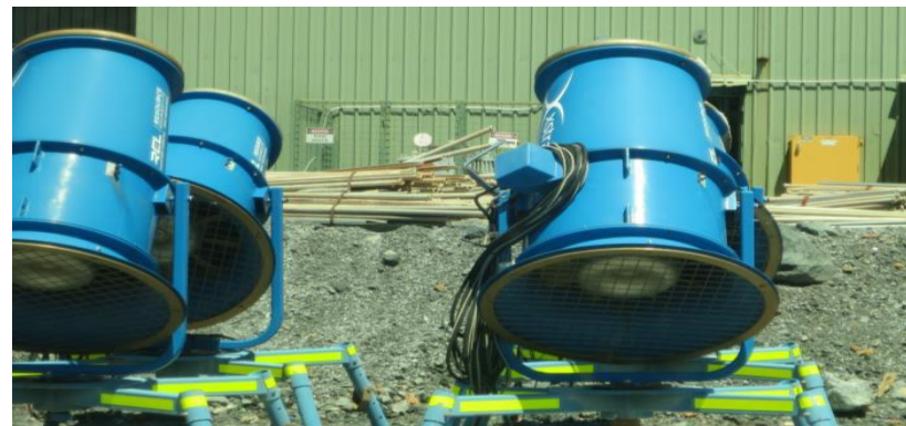
Water evaporation fans
