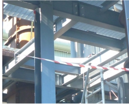
Detail of the support beams and cross members installed in Level 9 of the North Tower
