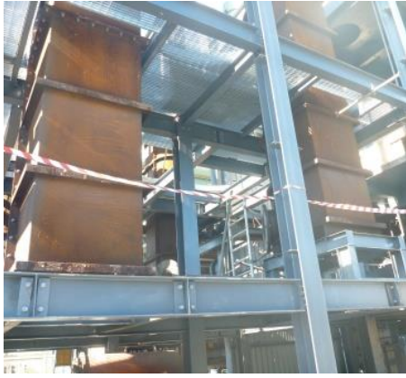
A completed section of the steel structure of RL9 which will support the G&M fluid beds
