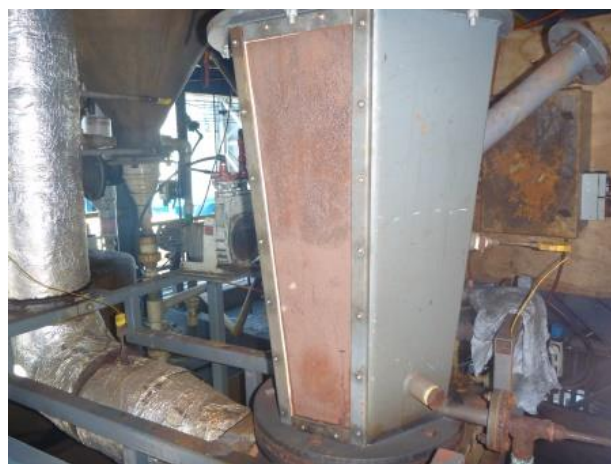
The fluid bed evaporator producing iron oxide/iron chloride pellets from pickle liquor and furnace dust
