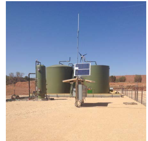
Production facilities on the Devon Bishop 1H Cline Shale well
