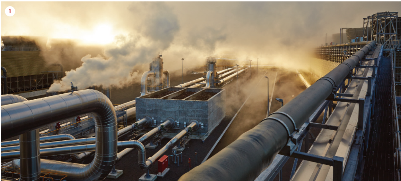
1. Te Mihi power station
