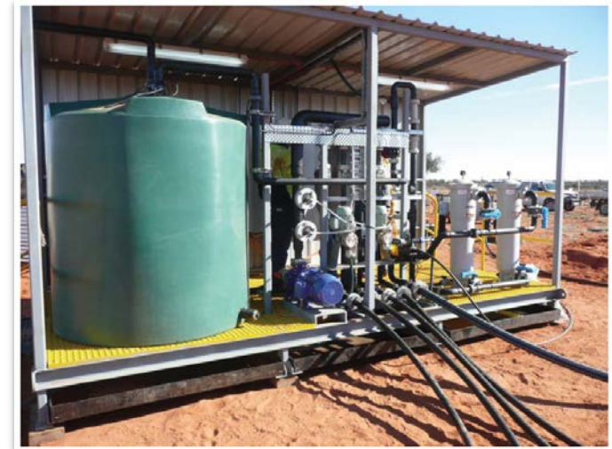
Example of FLT unit
