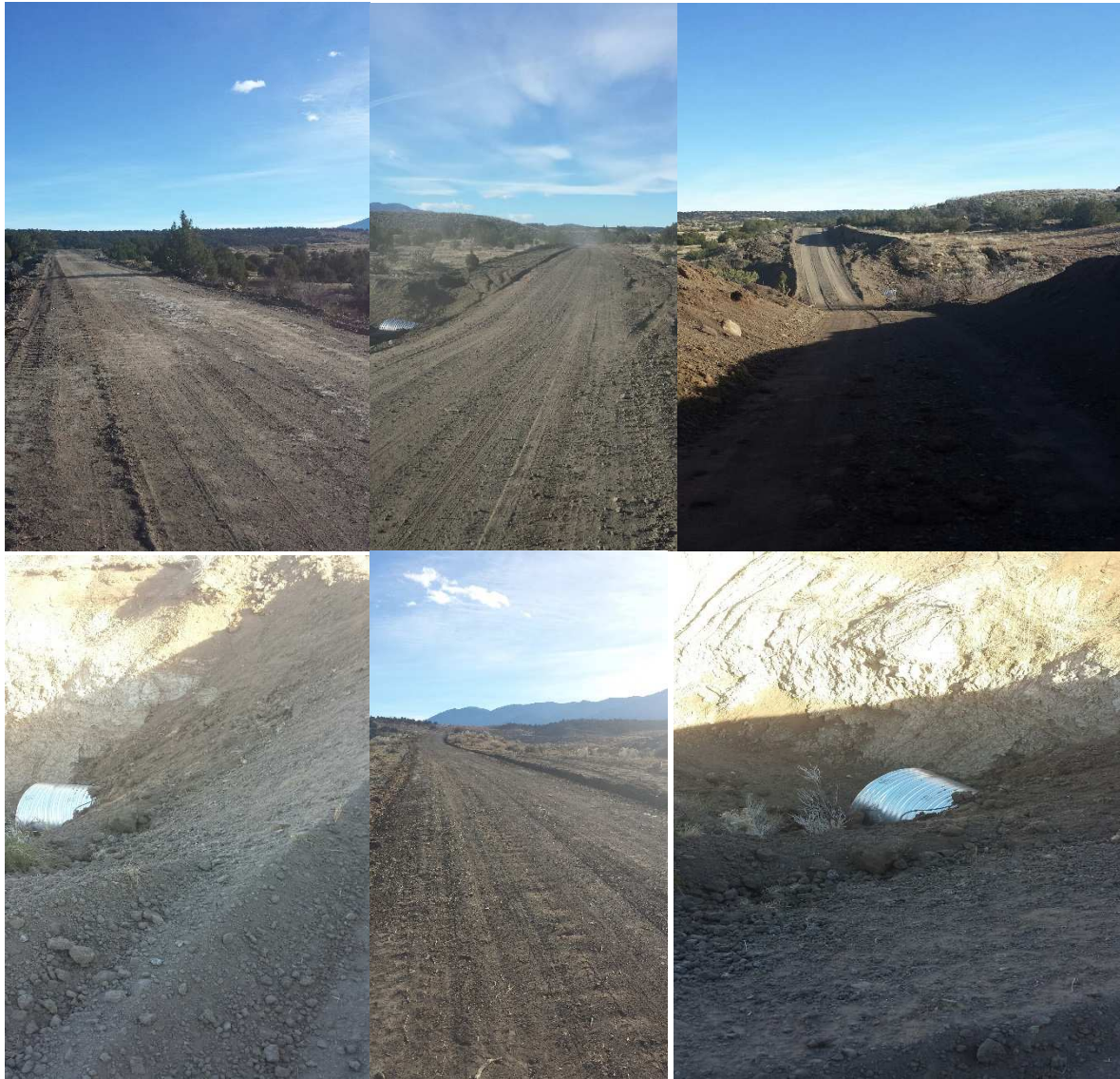
Pictures of the newly completed access road that allows access to six 640 acre one square mile tracts
