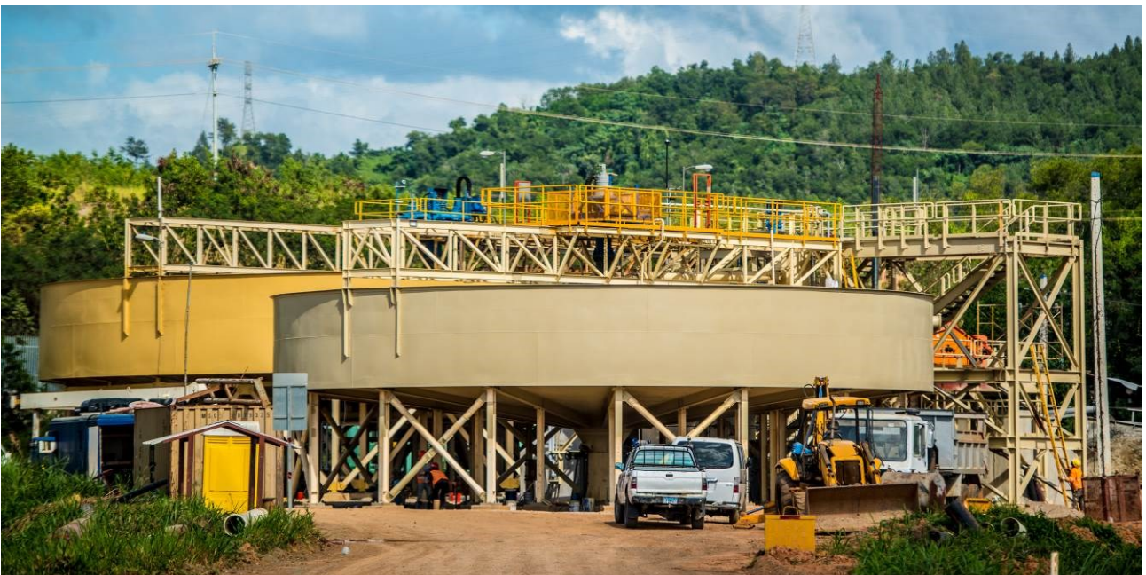
Processed Tailings Thickener & Plant Feed Thickener
