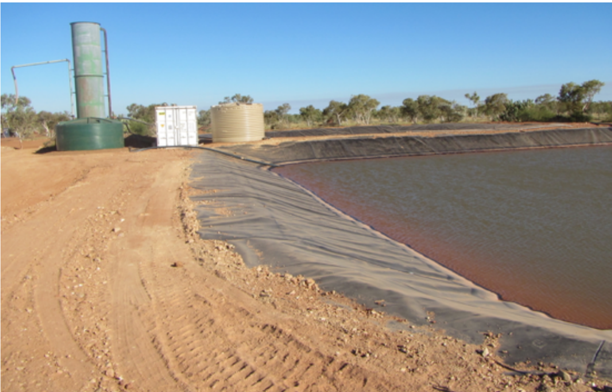
Process Water Facility
