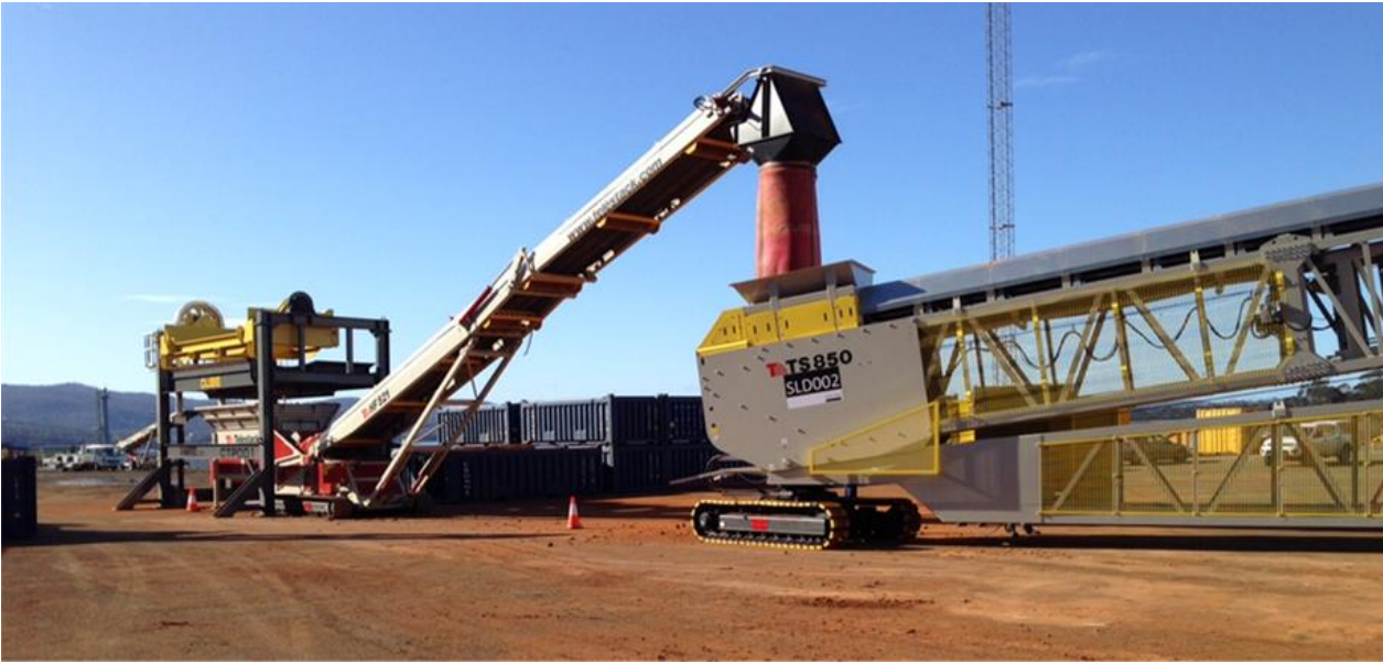
Unload tipper for discharge from rail into radial stacker at Bell Bay Port
