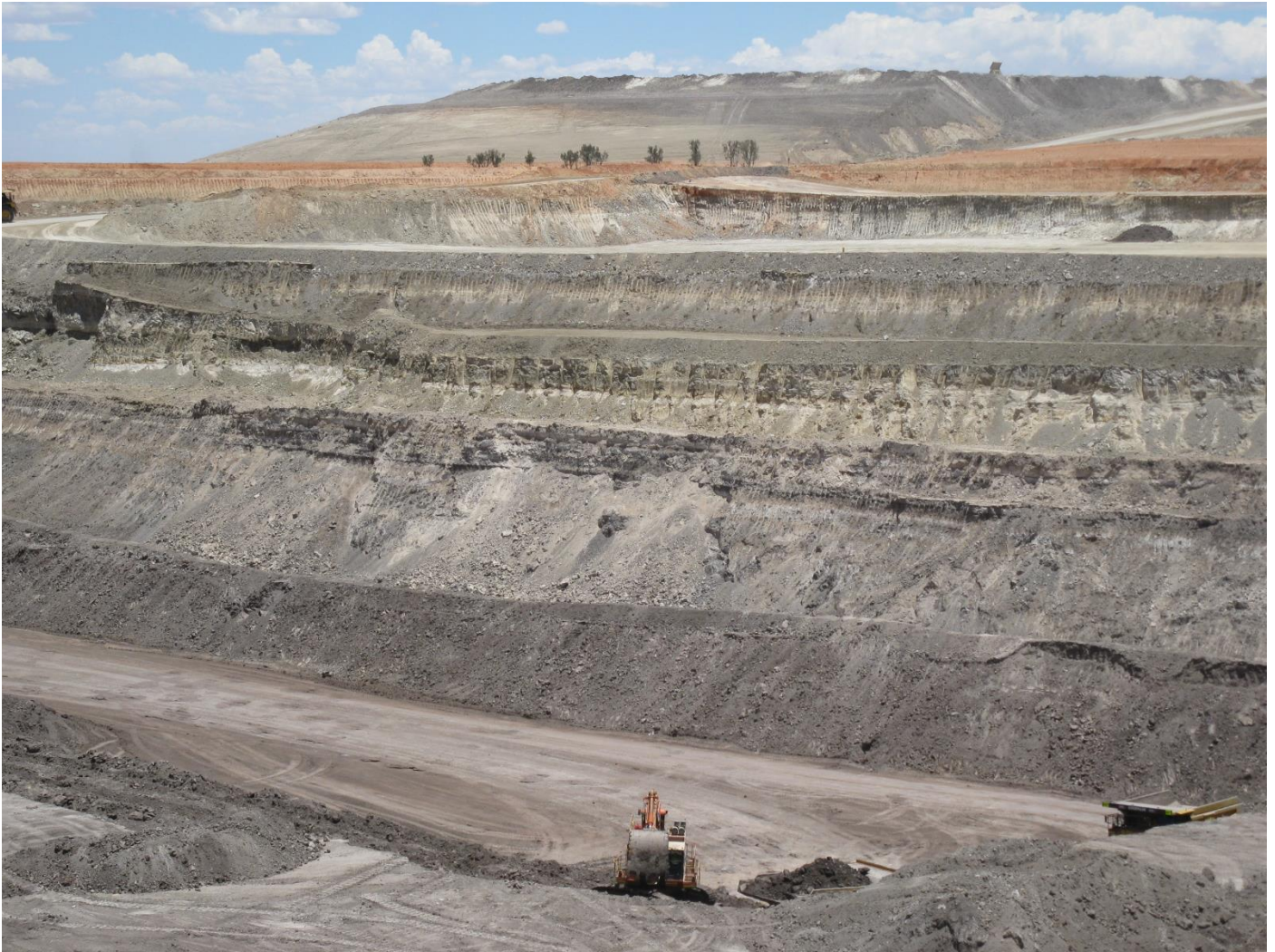
Portia open pit and waste dump as of last week (looking southwest). The ramp for the interim open pit (to be steepened) lies in the foreground.
