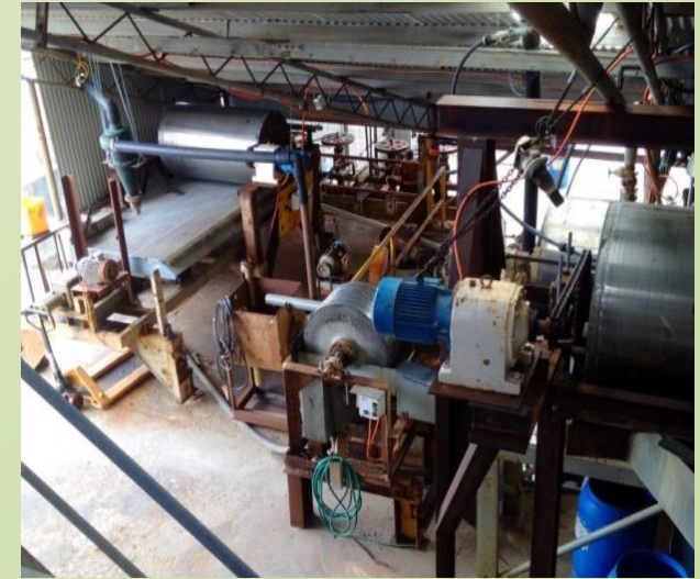
Granville Tin Project - Processing plant
