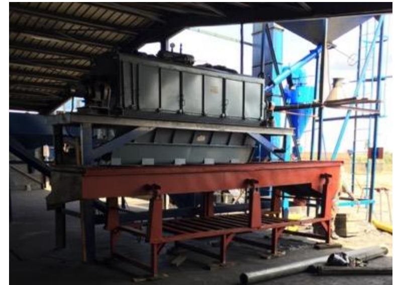
Improvements in action: Vibrating magnetic separator recently installed at Graphmada
