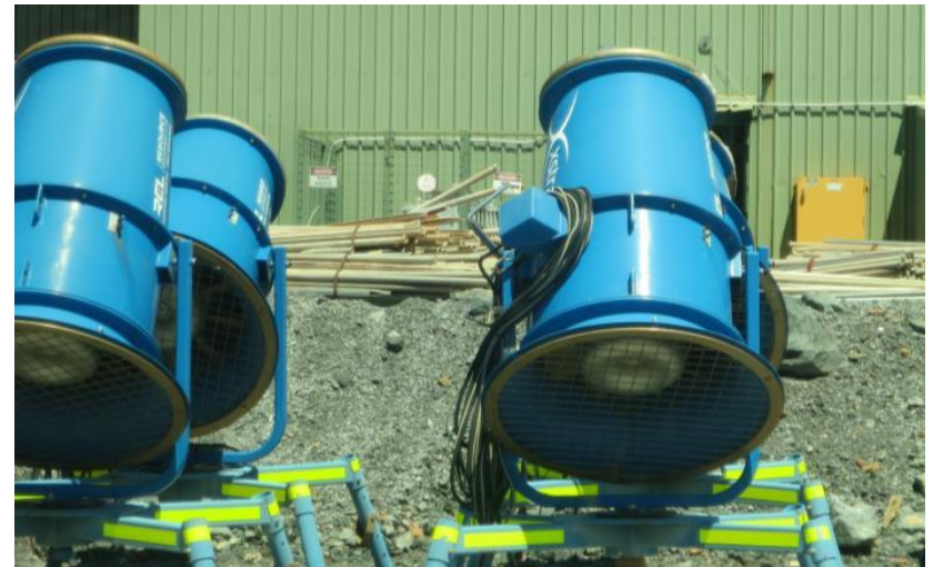
Water evaporation fans
