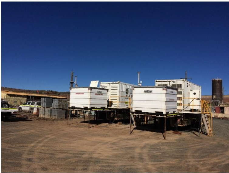
Photo 9: Diesel generators installed
