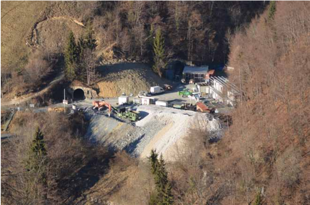
Figure 3: Gorno Zinc Project, showing recent development and rehabilitation at the Ca Pasi entrance to underground workings
