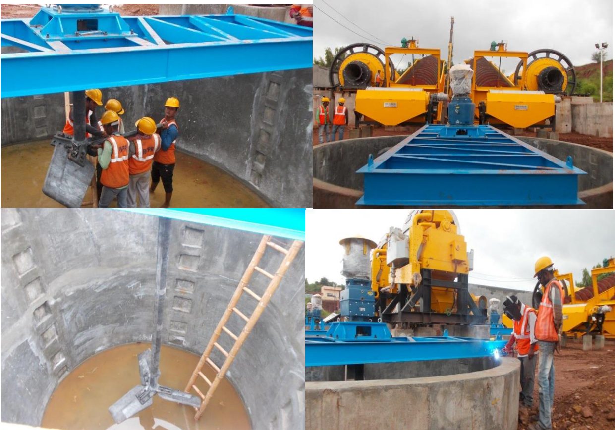
Equipment prepared for commissioning
