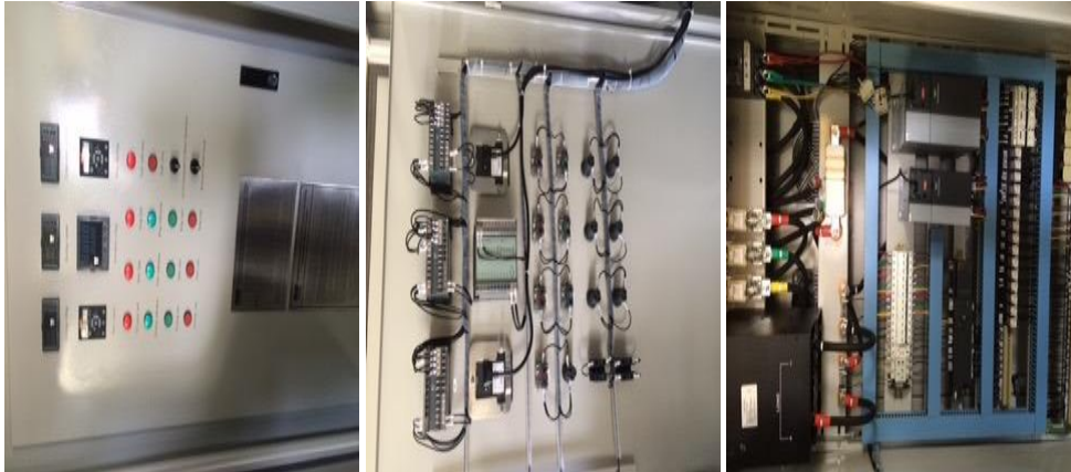
Magnetic separation equipment control panel post testing and ready for packing
