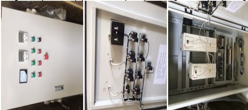
Water filtration equipment control panel post testing and ready for packing
